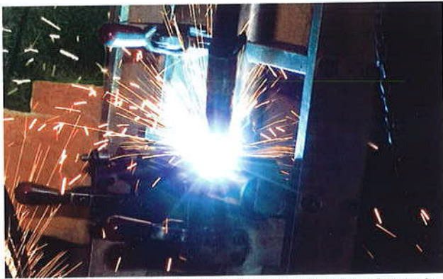
A variety of steel shapes are joined using the latest in welding technology to produce high-strength, durable structures that support heavy loads under many years of constant usage. Welding personnel and robotic welding processes are certified by an independent agency to ensure consistent quality.
