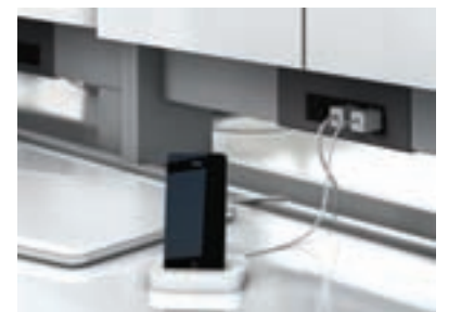
Power and data outlets are placed within arm's reach while an integral trough below the worksurface conceals excess cabling. Easy!
